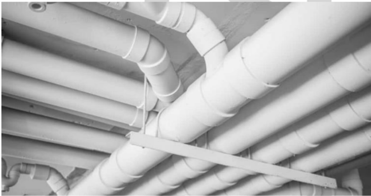
uPVC Pipe Work
